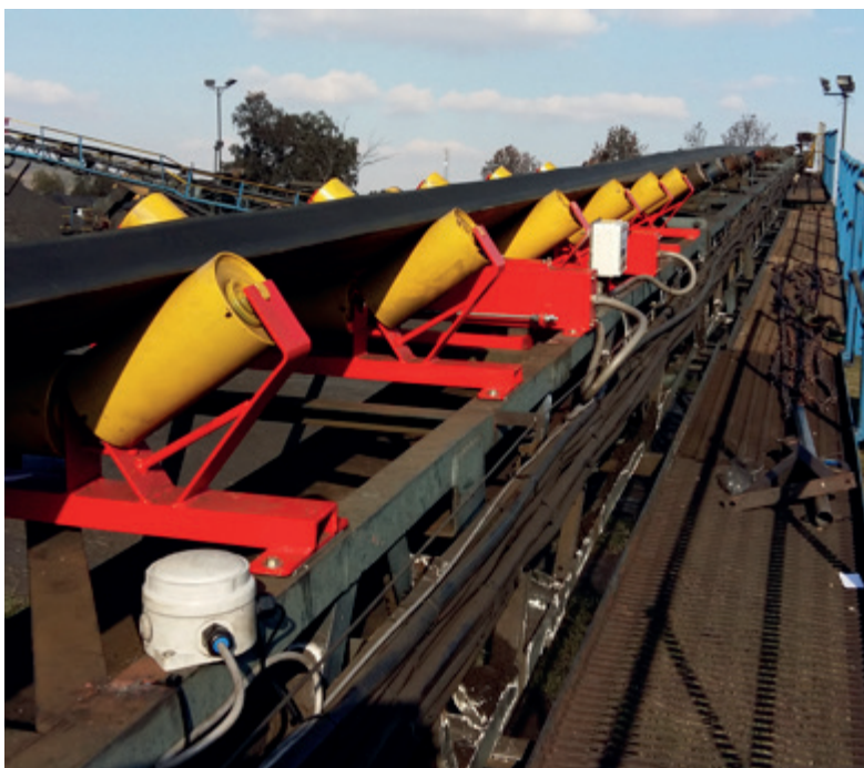
TYPICAL IN-SITU BELT SCALE ON PRODUCT FEED APPLICATION.
