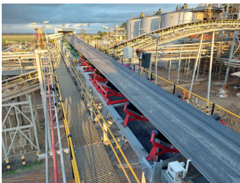
Sasco Belt Scale Installation in Ghana
