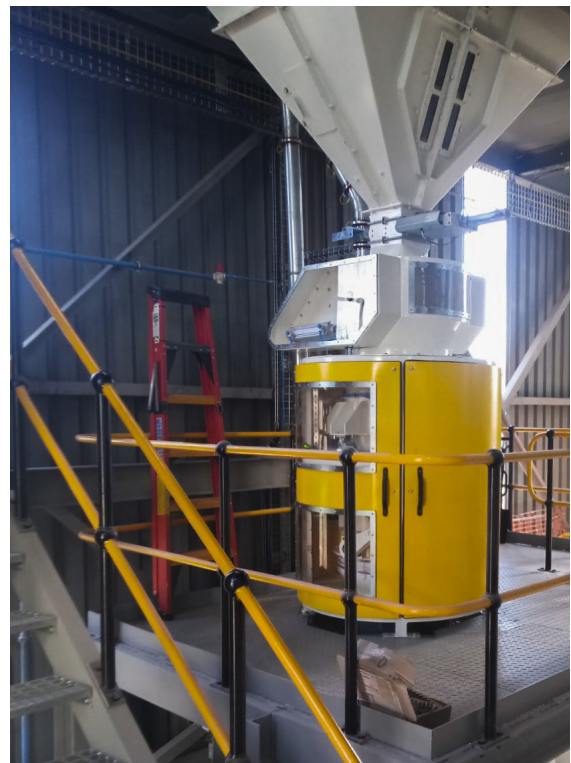
Sasco AGTW Installed
